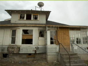
Open and/or unsecured structure(s). IPMC § 111.2
