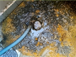
Improper maintenance for damaged sewer drainage system. IPMC § 506.2
