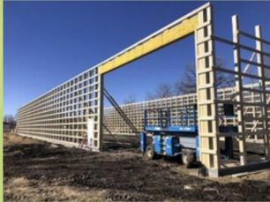
Construction without benefit of permits. KC Building Code Violation § 105.1
